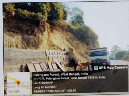
Structural measures taken to protect landslide areas, Algarah and its surroundings, Kalimpong district, West Bengal
